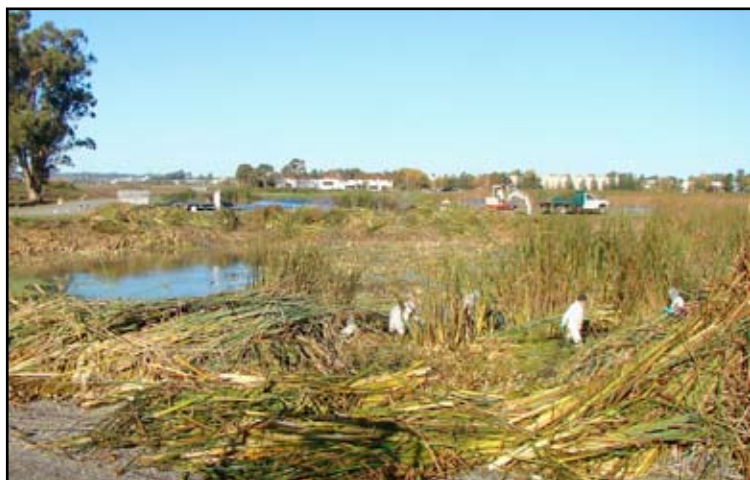
Figure 1. Workers remove excess Cattails during the draining of Pond A at Ellis Creek
